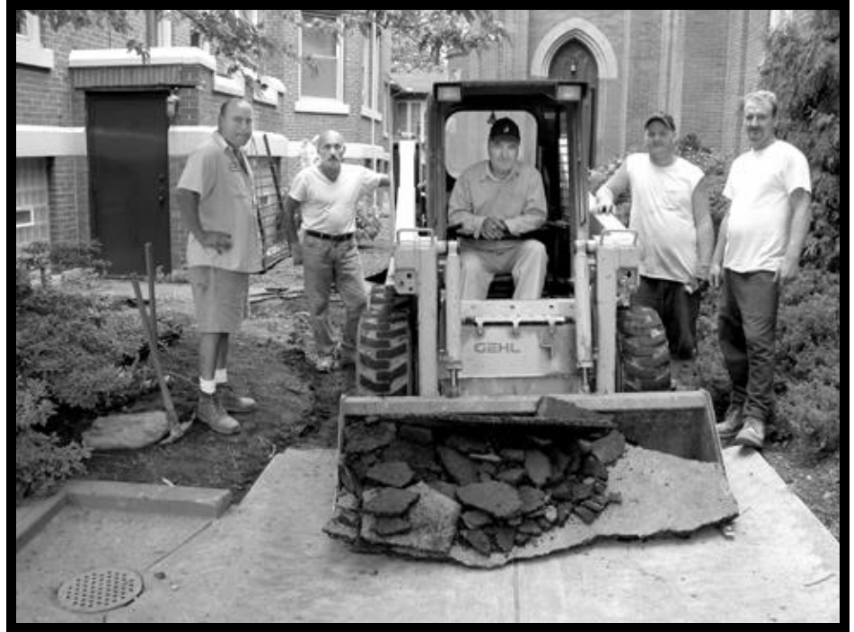
CECCHI CONCRETE CO. is donating all the concrete work for the walks in the garden area between the rectory and the church. The crew first had to dig up and remove all the old concrete and asphalt. Then Joe Calamante set the forms for the concrete which was poured and finished by the Cecchi Co. Pictured above from left to right are Rick Cecchi, Mark Cecchi, Lou Cecchi (sitting in the bobcat tractor and owner of the company) Keith Brown and Mark Gannon. Lou Cecchi is a member of the parish and graciously offered his assistance when he found out we needed this work to be done!
