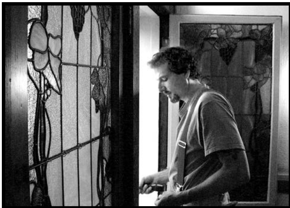
Getting Closer to Completion! A carpenter installs the restored stained glass windows in the stairwell to the Rectory's second floor.
