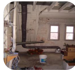
Attic with buckets catching rain drops!
