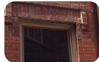
Deteriorating window lentil
