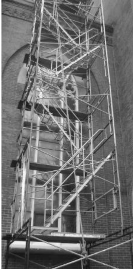
Scaffolding ascends the side of the church at the ramp door as the window frame is restored.
