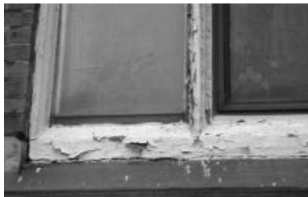
Peeling paint and loose wood endanger the exquisite windows.
